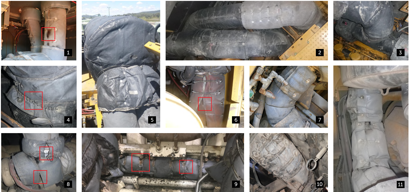
ABOVE Fix and refit blankets to avoid hot spots from gaps (1,6,8). Refit/replace stretched springs and loose tie-wire (4,6,8). Monitor and schedule replacement for wear (9), soot marks (2,3,8-11) and irreparable/loose fitments (8). Investigate burn marks for exhaust leaks (1,8).
